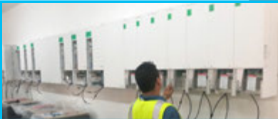
Puerto Rico Microgrids 100 schools are powered by Microgrids through Red Cross's community resiliency project Solution: microgrids using XW+ inverter / chargers, MPPT 60/80 charge controllers and other communication devices.
